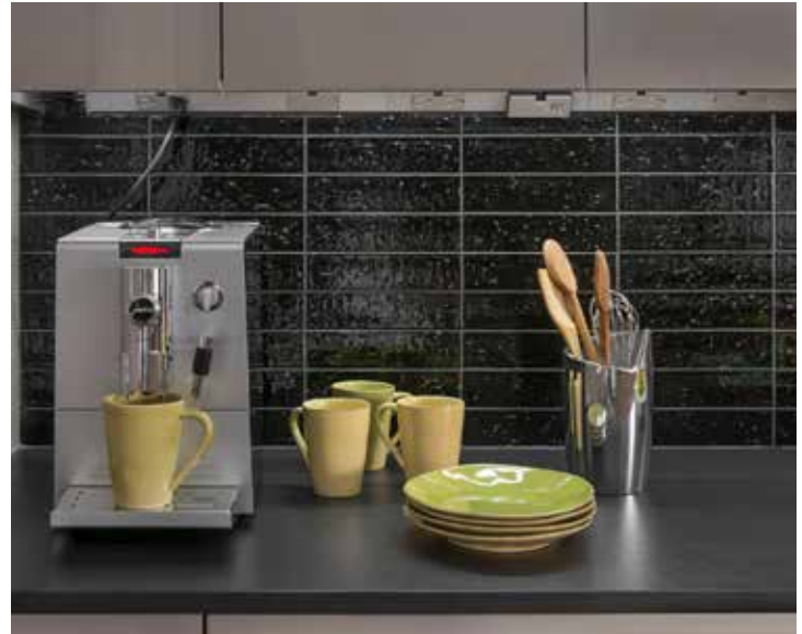
Under-Cabinet Lighting System installed in a kitchen.
