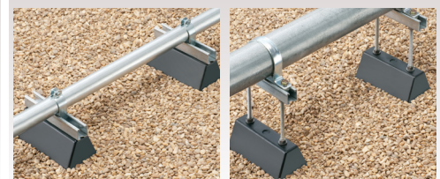
Raceway raised 12" above the roof
