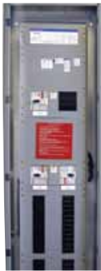
Wall-mount maintenance bypass panel
