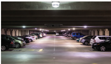
Before: Metal Halide Lighting
