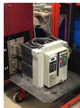
Primary Injection Testing
