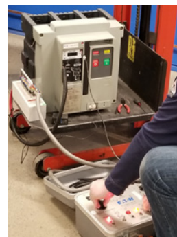
Secondary Injection Testing
