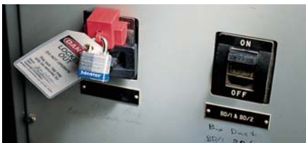
Oversized Breaker Lockout Device
