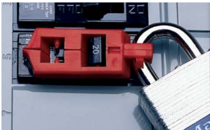
Single Pole Circuit Breaker Lockout
