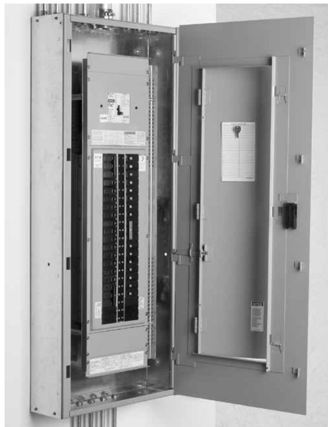
Trim Hanging on Surface Mounted Box
