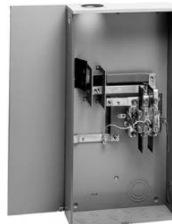
320 Ampere Lever Bypass Meter Socket
