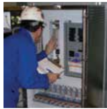
Control and Monitoring
