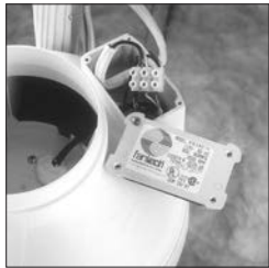
Romex wiring – Top View
