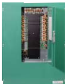
Lighting Control Panel
