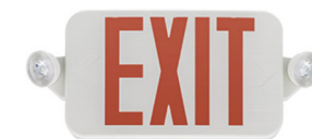
Emergency and Exit
